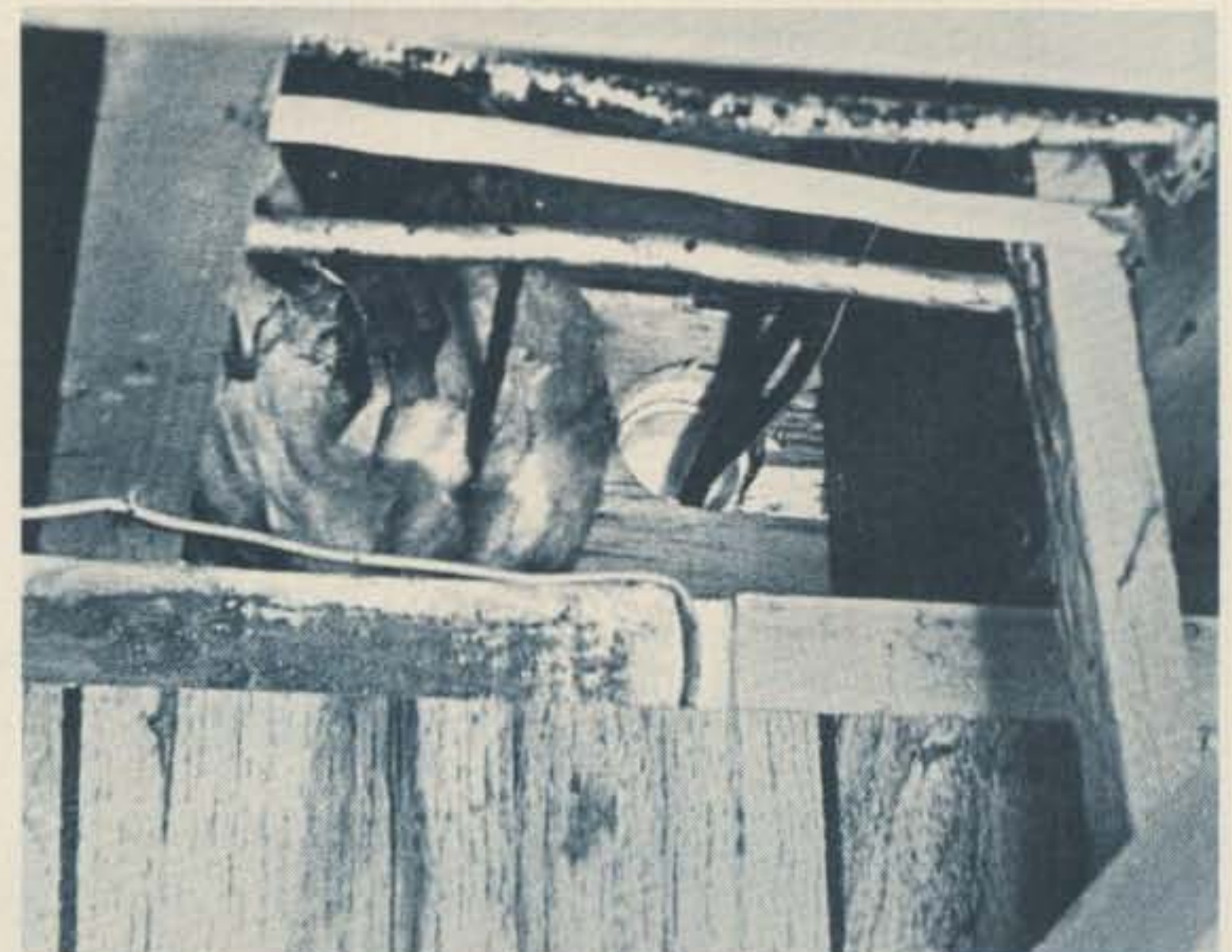
Inside-of-house view of the 90° elbow and the cables routed through it into the house.
